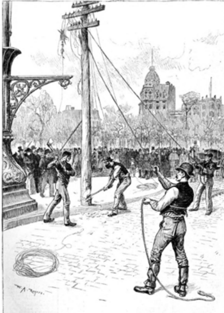
Removing the telegraph poles in Union Square, New York City” Quelle: Harper’s Weekly Nr. 33, S. 337.
